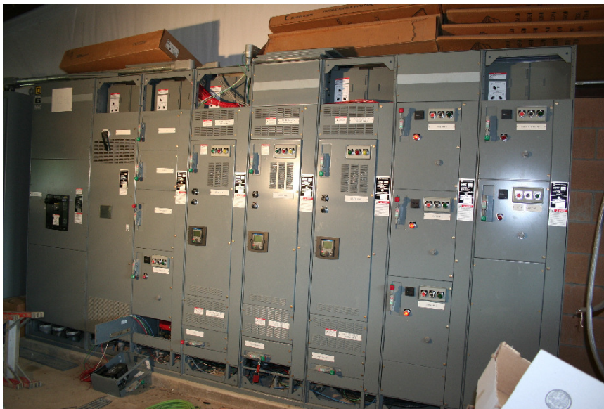
Electric Control Center
