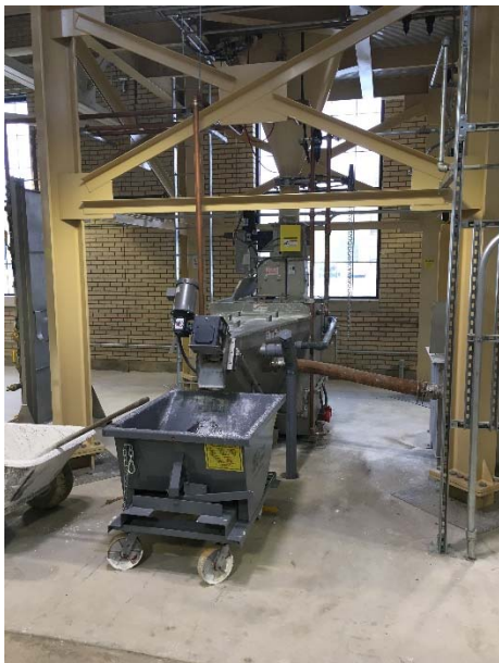
Headhouse Lime Slaker – View 1
