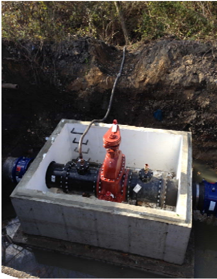
Valve Replacement Project Phase III Site F (Main and 5 th St) Niles 20-inch Valve and Vault
