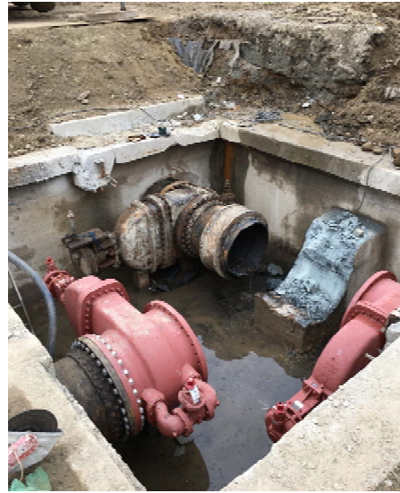
Valve Replacement Project Phase III Site L & M (Salt Springs and Bridge) 42-inch Valve and Vault
